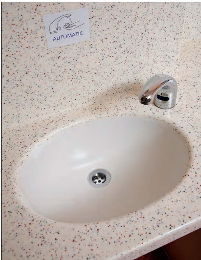
A separate wash-hand basin should be provided for use by staff conducting decontamination. This basin should be distinctly separate from the sinks used in decontamination
